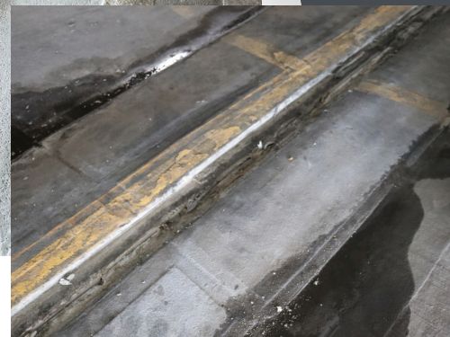
Deteriorated expansion joint area prior to rehabilitation.
